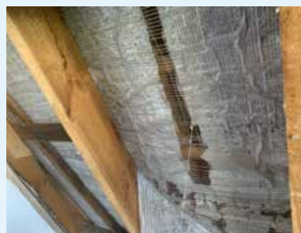
Fig. 12: Old, damaged underlay membrane (with scrim reinforcement) – outgassing of volatile plasticisers has led to significant embrittlement.
