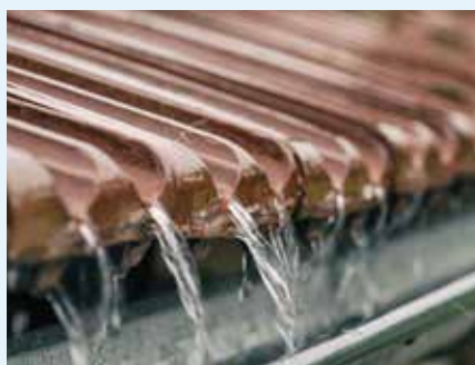
Fig. 7: Protection against the elements is mainly provided by the roof covering on the finished roof. However, water may still breach the roof covering in the case of driving rain, for example.
