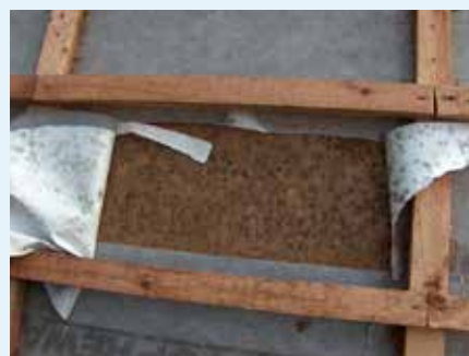
Fig. 30: Mould infestation underneath a microporous underlay membrane – the wood fibreboard underneath the membrane has become damp due to weak passive moisture transport, thus providing favourable conditions for mould growth.
