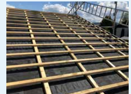
Fig. 4: Roofing underlay with sealed overlaps and joints and with nail-sealing tape (not visible here) to seal perforations.
