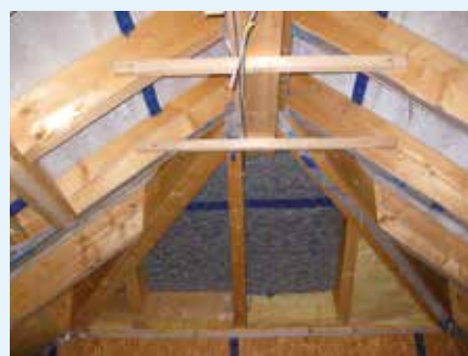
Fig. 31: On this project, monolithic SOLITEX membranes (hip roof at the centre of the photo) and microporous membranes (main roof surfaces on left and right) were installed side by side; under identical conditions, the microporous membrane has a water film, the monolithic membrane remains dry.
