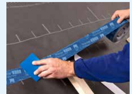
Fig. 5: Obligatory measures when using roofing underlay membranes as a temporary covering: Taping of seams and joints with adhesive tape or integrated self-adhesive strips.
