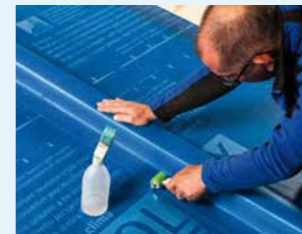
Fig. 18: Welded underlay membrane with enclosed counter batten – this represents the highest category of additional rain-protection measure; it offers very high protection against rain, even at particularly low roof pitches.
