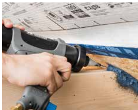
... joints at double collar ties that are difficult to access,
