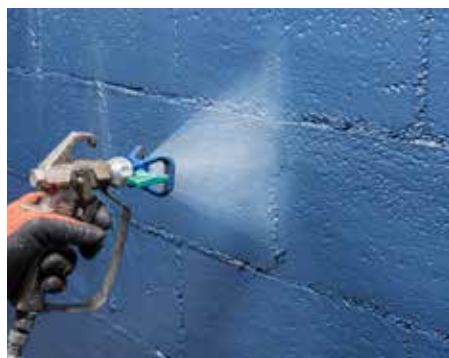
... unplastered walls, and
